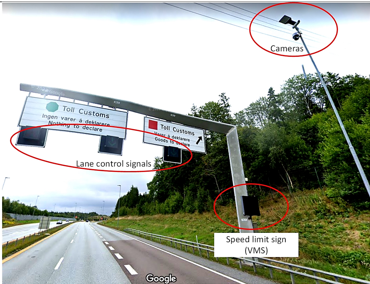
Figure 10: Example on Roadside equipment at Svinesund Customs, Norway (picture source: Google aps/Streetview)
