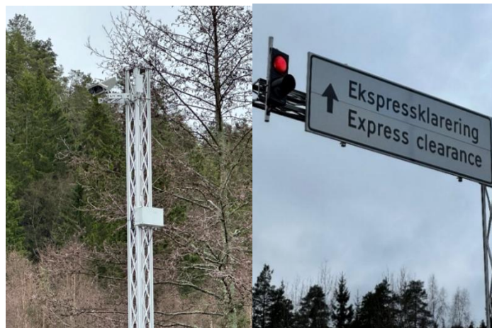
Figure 2: ANPR-camera at the Svinesund customs station and the light signal at the Digitoll express clearance lane (B in Figure 1).
